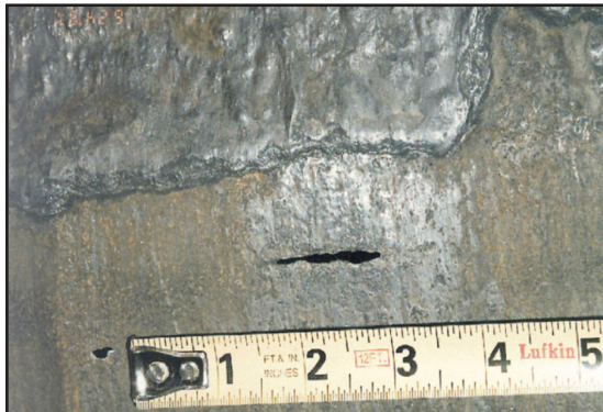
Abrasion and corrosion caused through wall damage in many areas of the silo
