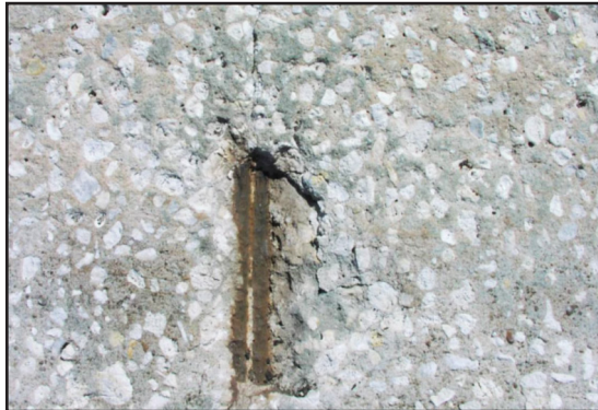
Corroded concrete with exposed rebar
