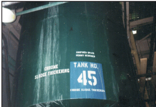
Waste treatment tank
