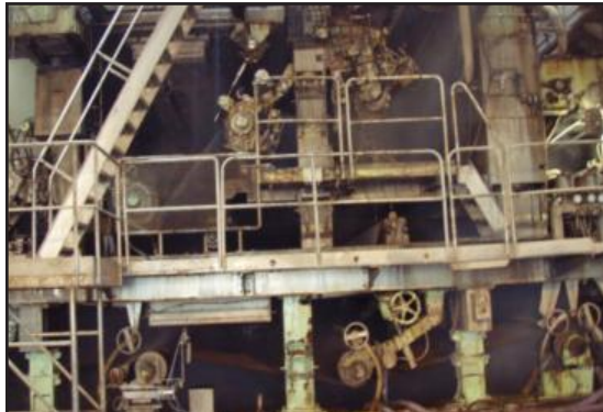
Corroded structure of old paper machine
