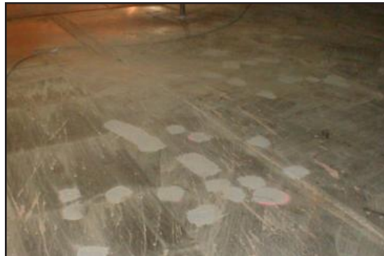
Severe pitting corrosion found under the existing coating repaired with ARC 858
