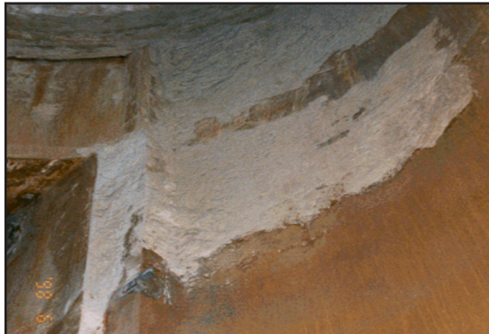
Severe corrosion inside the stack
