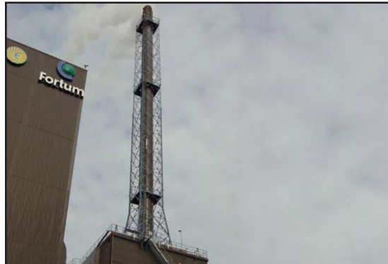
The flue gas chimney at wood and peat burning power plant
