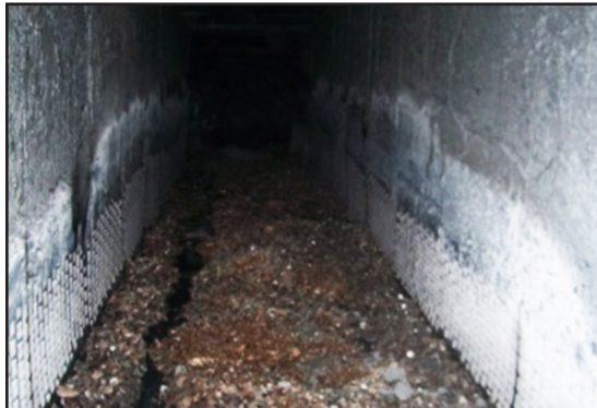
Discharge flume with damaged tile/rubber liners
