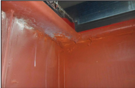
Original coating typically started to fail within 12 months of application
