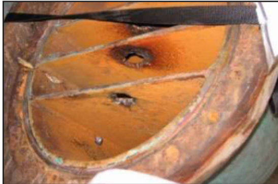
Corroded divider plates
