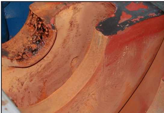
Eroded and corroded pump volute
