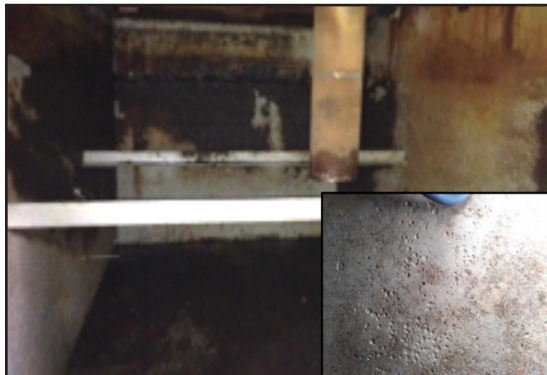
Heavy pitting corrosion in glycol water tank
