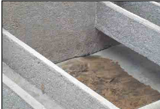
Drained sand filter vessel
