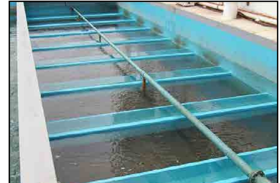
Sand filter in service
