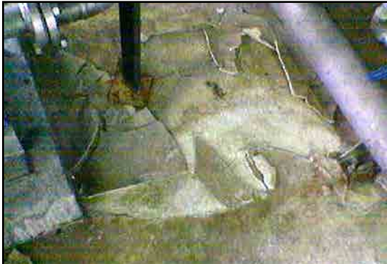
Delaminated glass matt polyester
