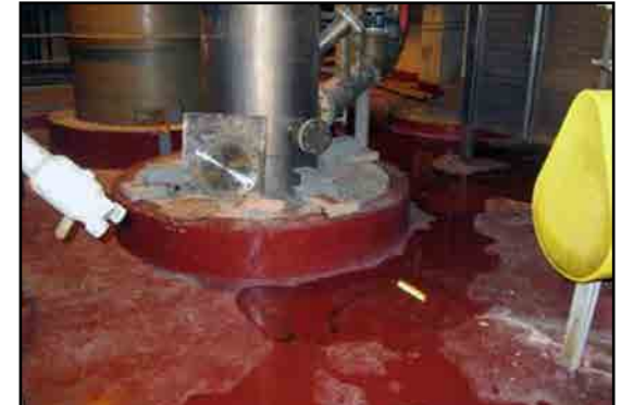
ARC NVE VC in service
