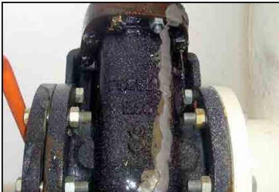
Valve leakage plugged
