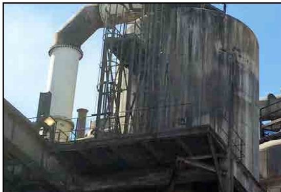
Flash cooler with exhauster
