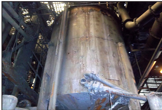
Tank in operation in highly corrosive environment
