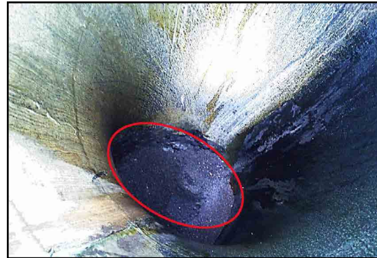
Dark scale formation on unlined section
