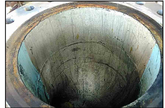
ARC S5 prevented corrosion and scale formation after 27 months
