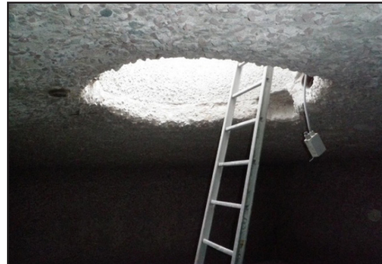
Surface of wet well was high pressure cleaned and abrasive sweep sandblasted.
