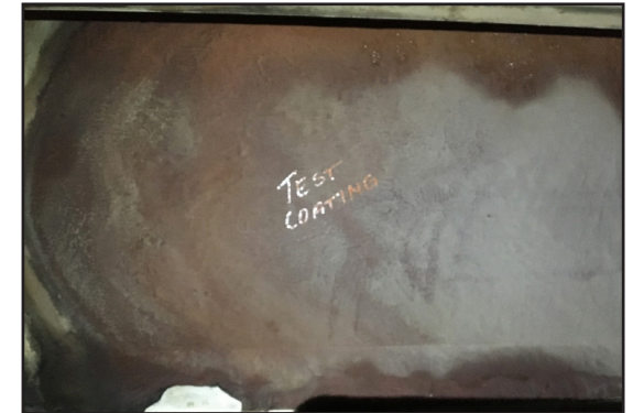
Test area of duct after nine months in service.
